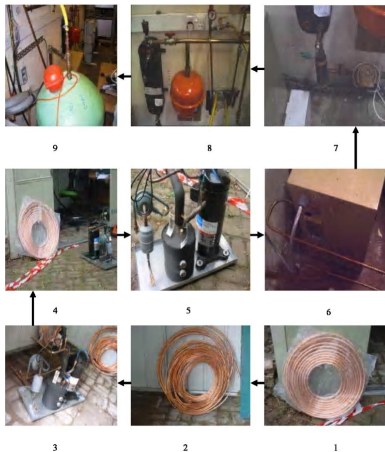
Figure 4. Showing preparation of coils (1-2), installation of heat pump (3-6) and connection of water supply system (water pump, flow metre, expansion valve and the boiler) (7-9)
